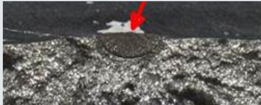
Photo of a crack after crack-opening, found during maintenance inspection. Crack depths 0,75 mm
