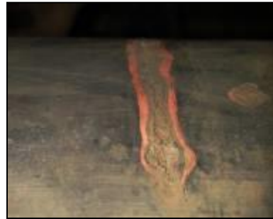
- Deep Corrosion Pit
